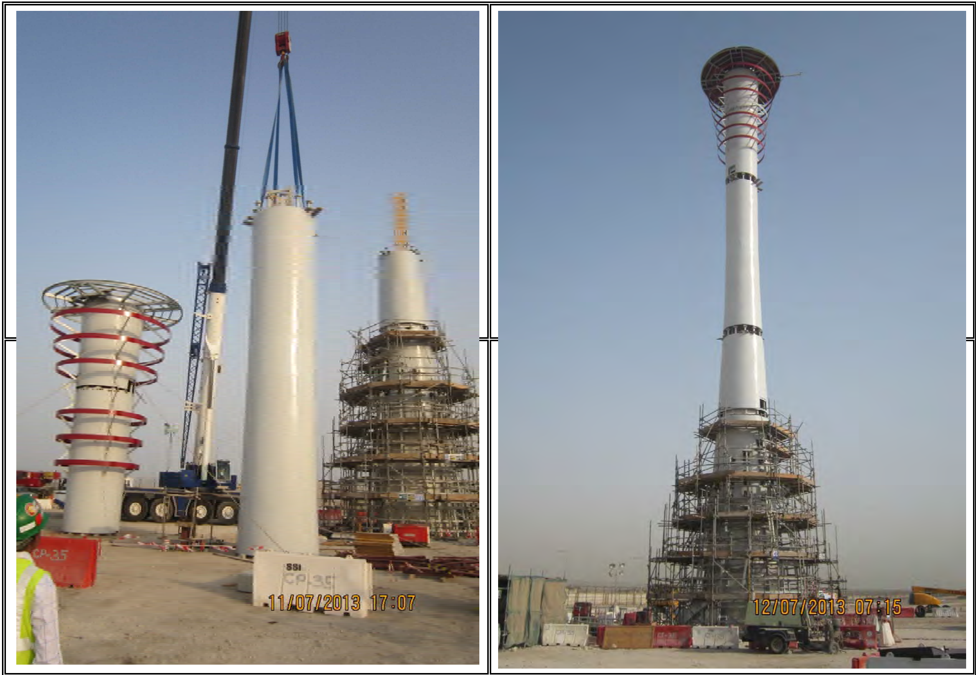
35 & 40 M RADAR TOWERS IN NDIA
